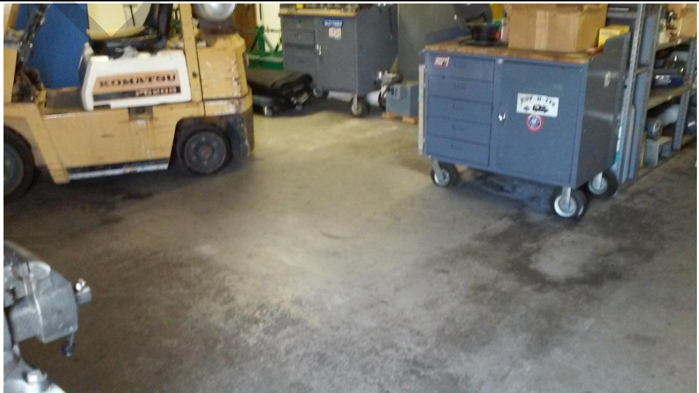
Photo 3 – The two concrete patches (center and lower right corner of the photo) were from a former waste-oil UST and two former hydraulic hoists. Located in the mechanical building.
