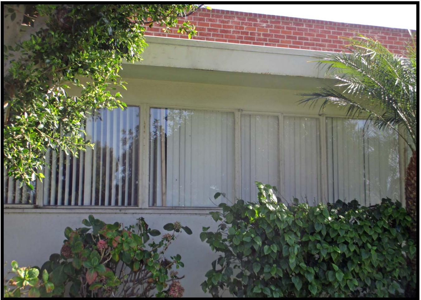
Detail of Fixed and Casement Windows on Western Elevation, Panama Street (SSE)
